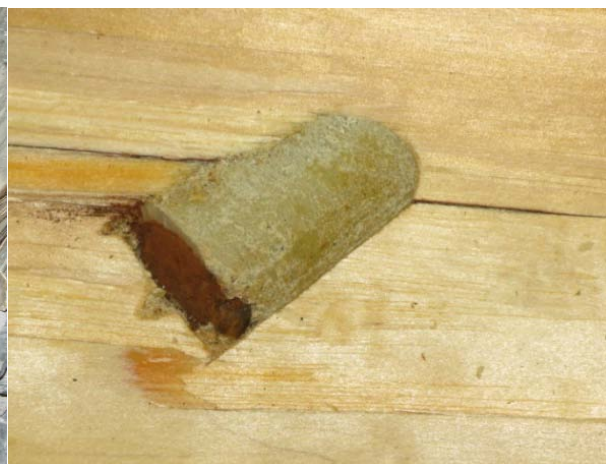
Fig. 11. The bottom end of the glued-in bar in wood after ten years outdoor condition and fatigue tests.
