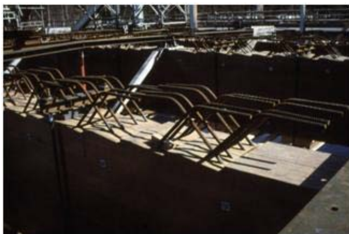
Fig. 5. The connectors and notches of the timber girders in the deck of the Vihantasalmi Bridge.
