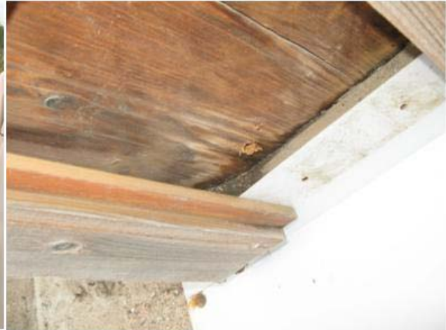
Fig. 17. Water pocket and crack at the end of the inclined load-carrying member.
