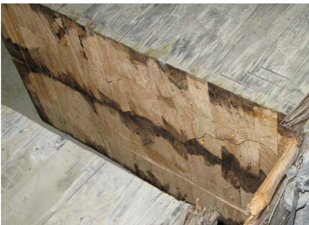
Fig. 10. Cross-section of the test beam after ten years outdoor condition and fatigue tests.
