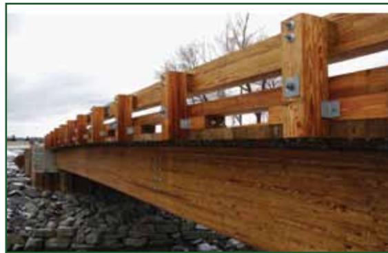
A two lane, 87-foot glulam girder bridge designed to meet AASHTO HS25 live loading.
