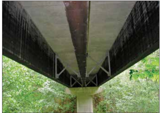
Example of composite timber girder–concrete deck bridge (Lola Coombe, USDA Forest Service).
