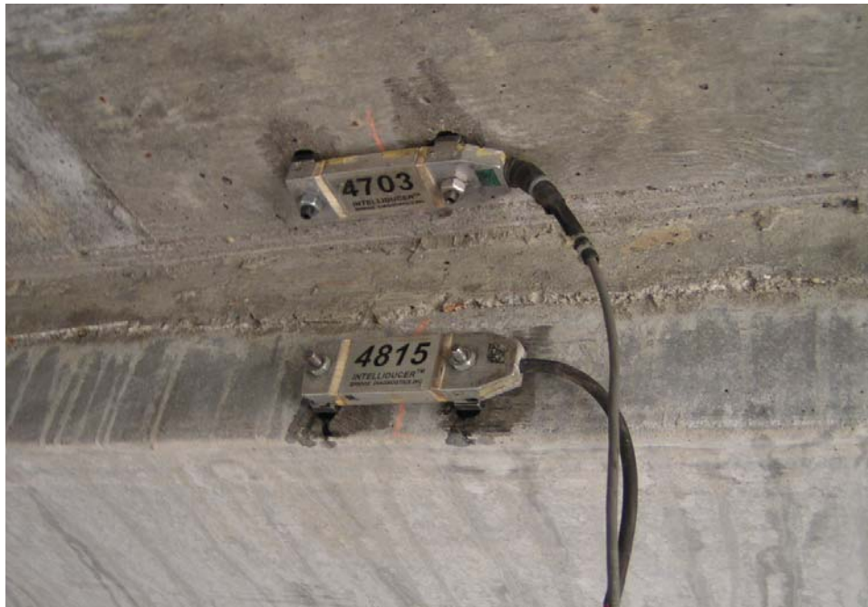
Figure 4.25. BDI strain transducers attached to concrete.
