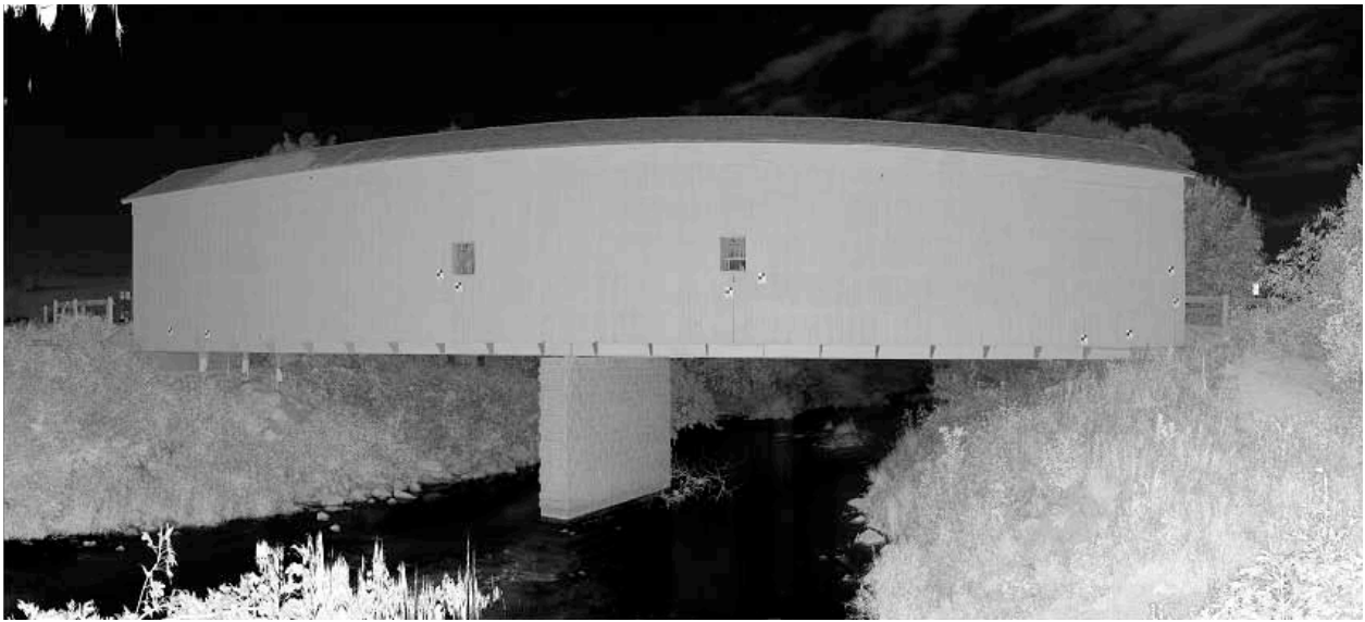
Figure 3B.-- A parametric picture of the outside of the Zumbrota bridge created from a single exterior scan (figure 3A) processed with Faro Scene software.
