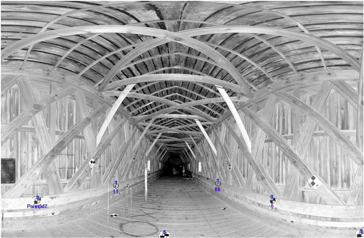
Figure 4.--A parametric picture of the inside of the Zumbrota bridge created from a single exterior scan processed with Faro Scene software.
