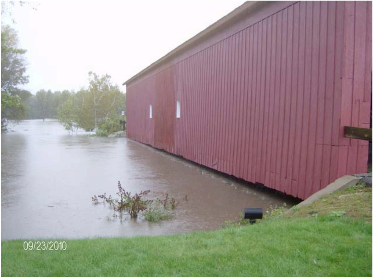
Figure 17.--Zumbrota covered bridge on September 23, 2010 during flooding on the Zumbro River (Photo courtesy of fox9.com).
