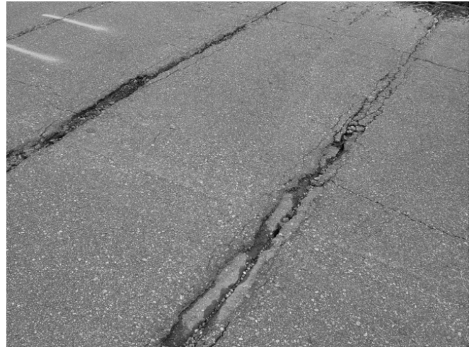
Figure 7. Butler County Bridge wearing surface deterioration.
