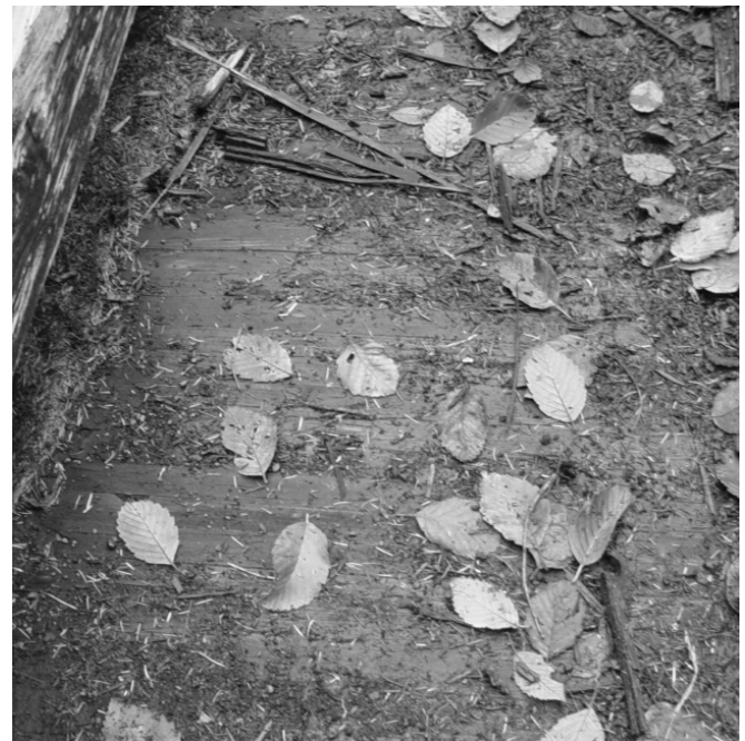
b. Exposed deck panels due to asphalt deterioration. Figure 4. Camp Creek Bridge wearing surface in 2002.
