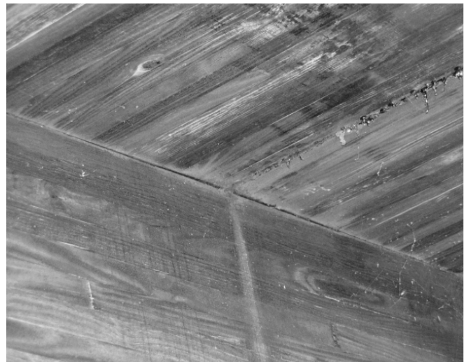
Figure 8. Cupping of deck panels on the Butler Co. Bridge.
