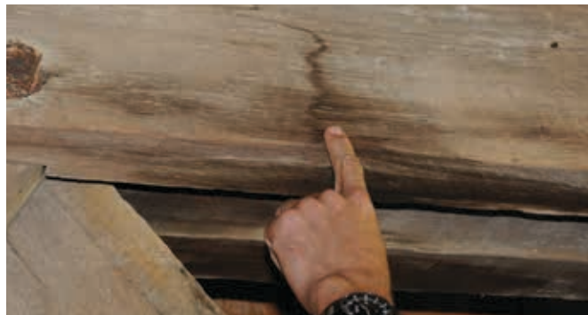
Figure 10.1—Indication of a water exposure event. Note the single color of stained material. If this were from multiple wetting events, multiple colors or bands of stains would be evident.
