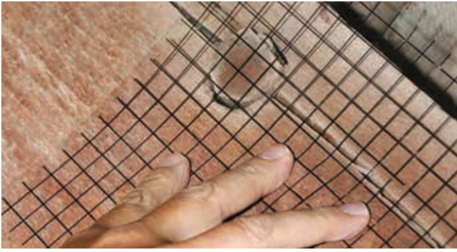
Figure 9.6—Example of using grid to establish the size of knot in bridge member. The measured knot in the example is 1-1/2 in.
