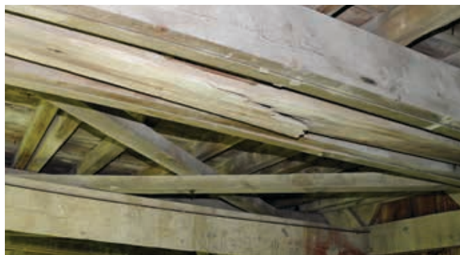
Figure 10.3—Failed load bearing member in need of replacement.
