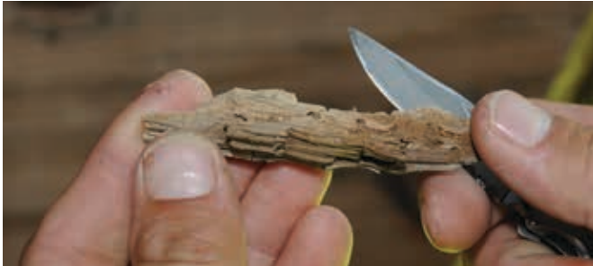
Figure 10.6—Example of a knife being used to probe wood: (top) Checking the soundness of wood and (bottom) an example of abrupt failure surfaces indicating decay.
