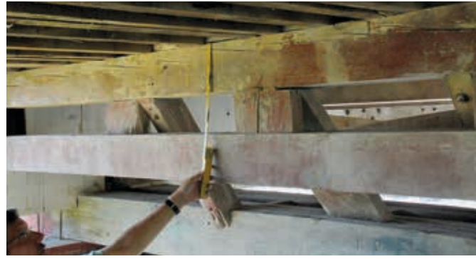
Figure 9.8—Example of using checking in a member to measure the slope of grain in bridge. The end of the scale points to the start of one check.
