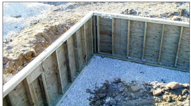
Figure 1—CCA is still registered for some residential applications, such as permanent wood foundations.
