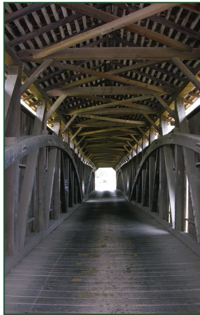
Pine Grove Bridge, located between Lancaster and Chester Counties in the Commonwealth of Pennsylvania, has burr-arch trusses in a two-span configuration.
