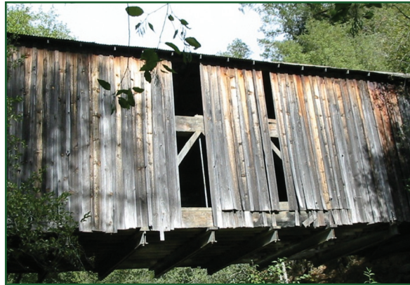
Vandalism exposed this bridge to rainfall
