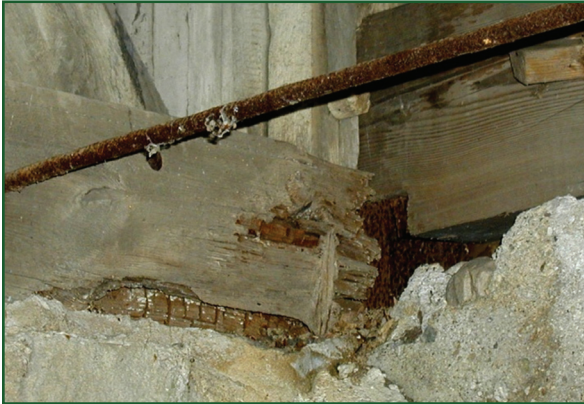
Decay at a covered bridge abutment that might have been prevented with field treatment
