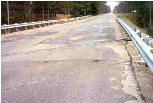
Figure 10—The La Chance bridge showing the asphalt wearing surface condition.
