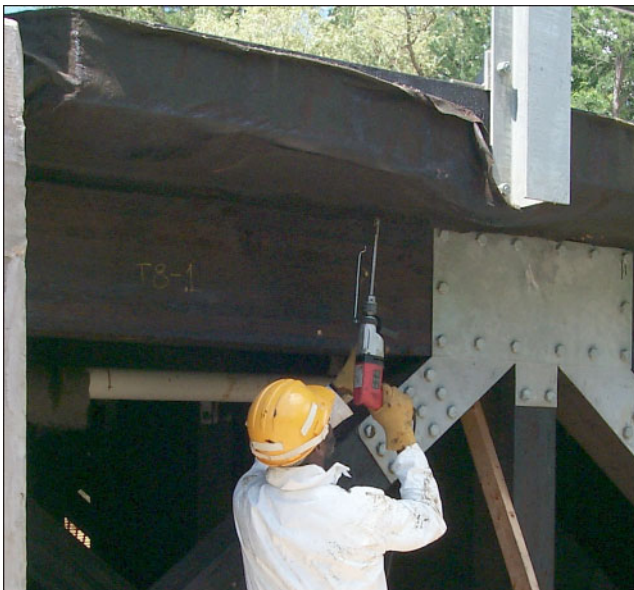
Figure 2—Removal of core samples from the La Chance bridge using an increment borer and hand drill.
