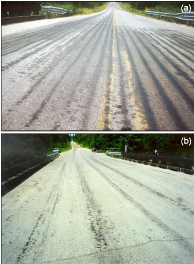
Figure 9—Creosote preservative visibly migrating upward through the asphalt wearing surface at the (a) Cruzen and (b) Cameron bridges.
