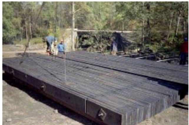
Figure 8—At the bridge site, the two deck sections were placed side-by-side atop temporary abutments located on the approach roadway.
