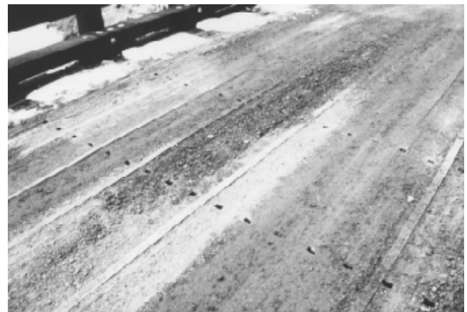
Figure 27—Debris accumulation on the bridge deck noted during condition assessment.
