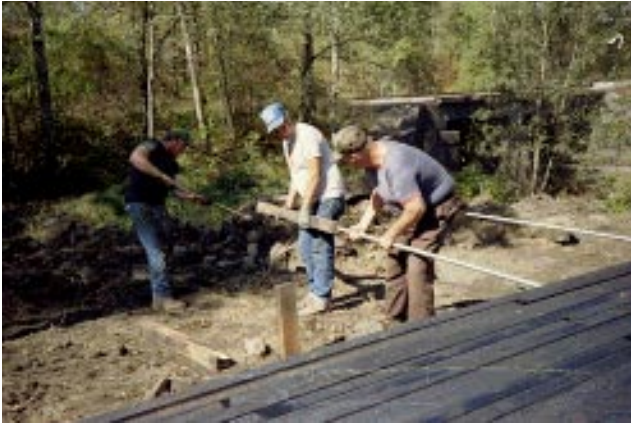
Figure 9—The temporary steel bars in the two deck sections were removed, and stressing bars were inserted through both deck sections.
