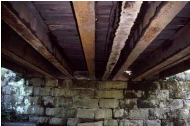
Figure 2—Original Hoffman Run bridge: (top) side view; (bottom) underside of bridge and abutment.
