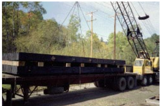
Figure 7—Two deck sections for the Hoffman Run bridge were transported from the treating plant to the bridge site on a flatbed truck.
