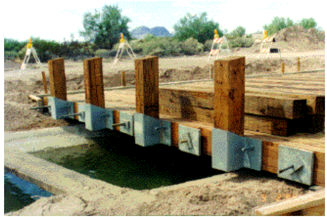
Figure 7—After deck assembly, steel post supports were attached to the deck and railposts were inserted.
