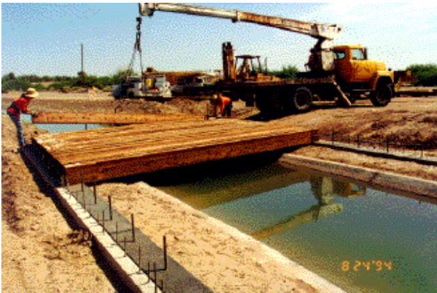
Figure 6—The Mohawk Canal bridge was assembled by a county crew: (a) Laminations were lifted by crane from the on-site storage location and positioned above the abutments. (b) Workers guided placement of laminations as they were lowered onto the abutments.
