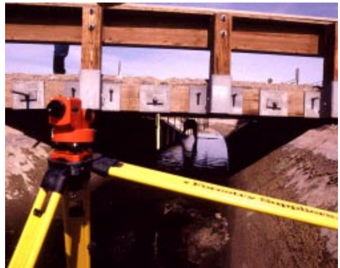
Figure 9—Load test deflection measurements were obtained by reading values with a surveyor's level from calibrated rules suspended from the underside of the deck.
