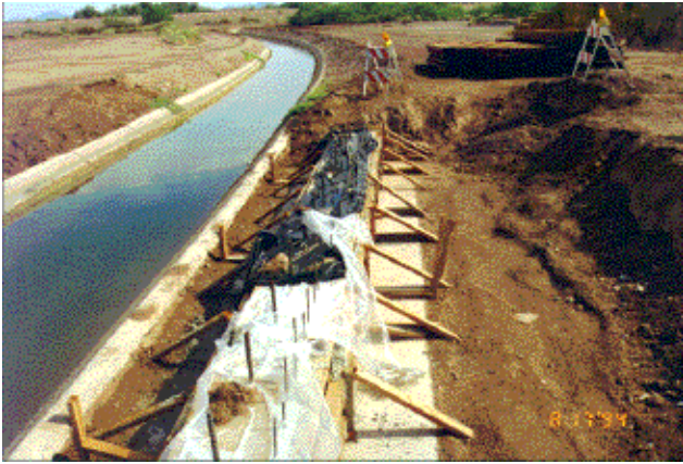
Figure 5—Construction of east concrete abutment and spread footing. The Douglas Fir glulam beams were stored on site for several days.
