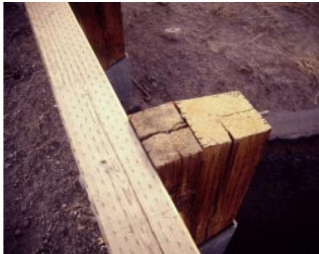
Figure 23—Severe checks and splits in railposts and spacer blocks noted during condition assessment.
