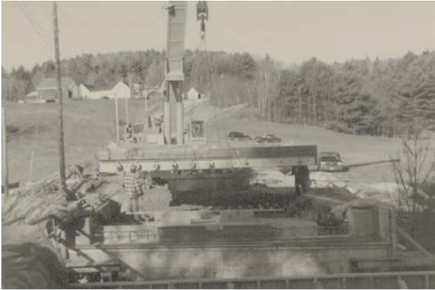
Figure 10—The entire deck was lifted from the temporary supports with a large overhead crane.
