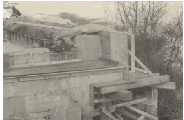
Figure 9—Prior to placing the deck, galvanized steel tie-down angles were bolted to the sides of the concrete cap of each abutment.
