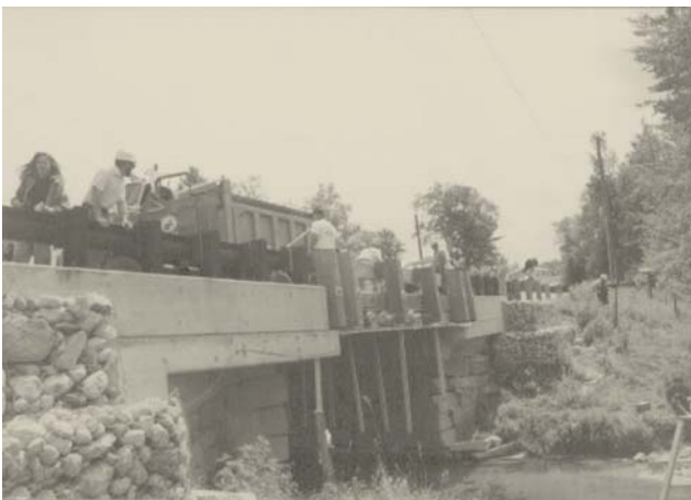
Figure 16—Load test 1. Bridge deflections were measured using a surveyor's level and rulers attached to stiff boards mounted to the underside of the bridge.
