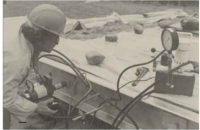
Figure 8—After the stressing system was installed, the bridge was stressed to the full design value.
