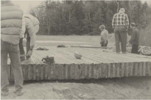
Figure 6—Preassembly of bridge at site on temporary timber supports placed adjacent to east bridge abutment.
