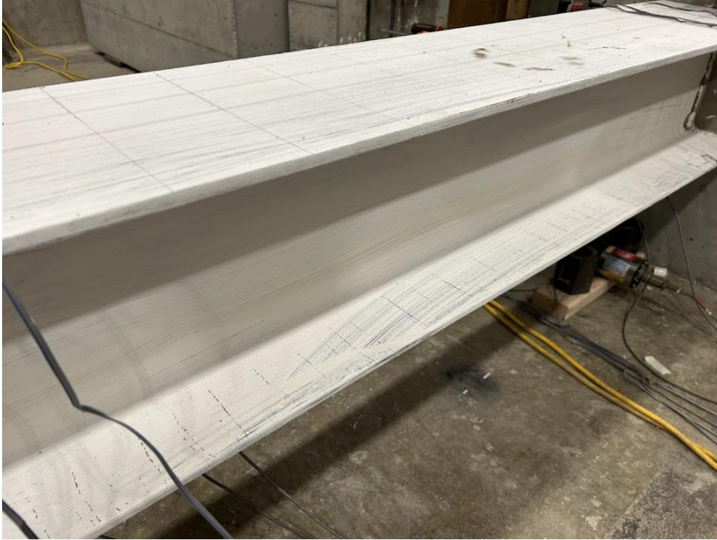
Figure 3-40. Transverse cracks in the lime wash on bottom flange – 2
