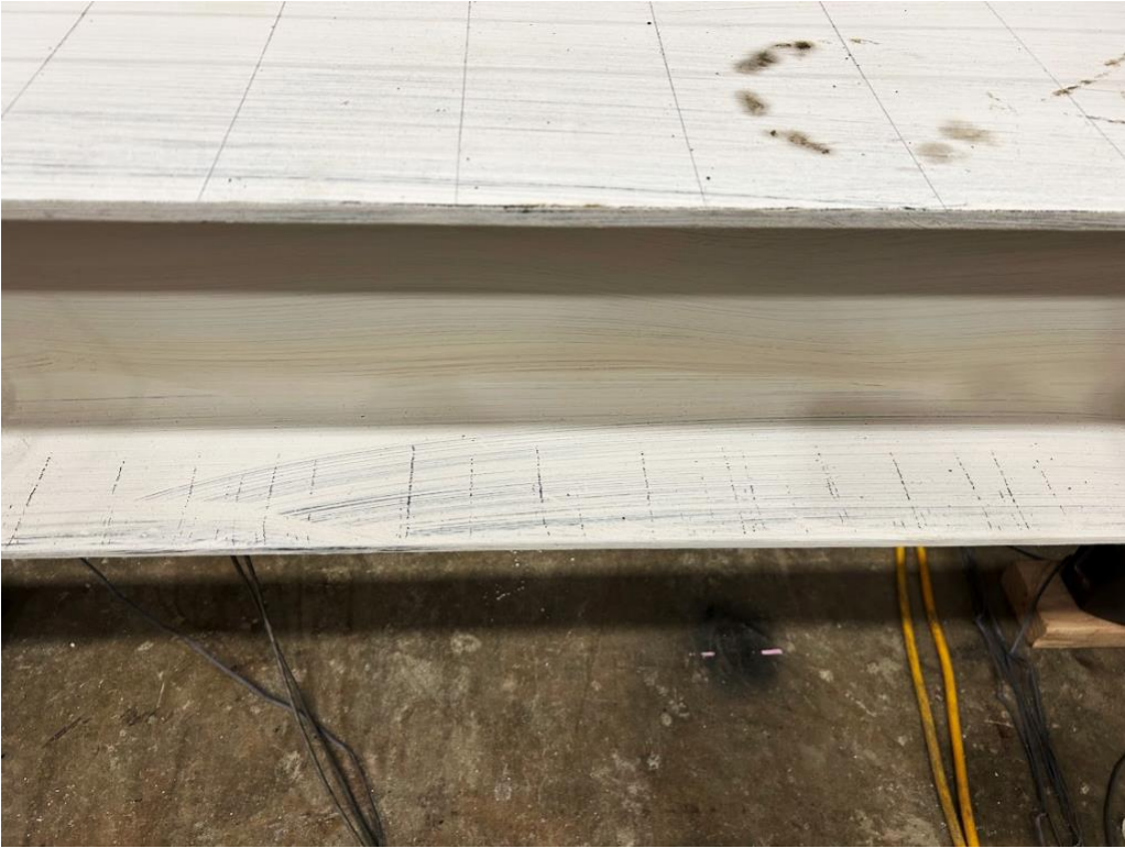
Figure 3-39. Transverse cracks in the lime wash on bottom flange – 1
